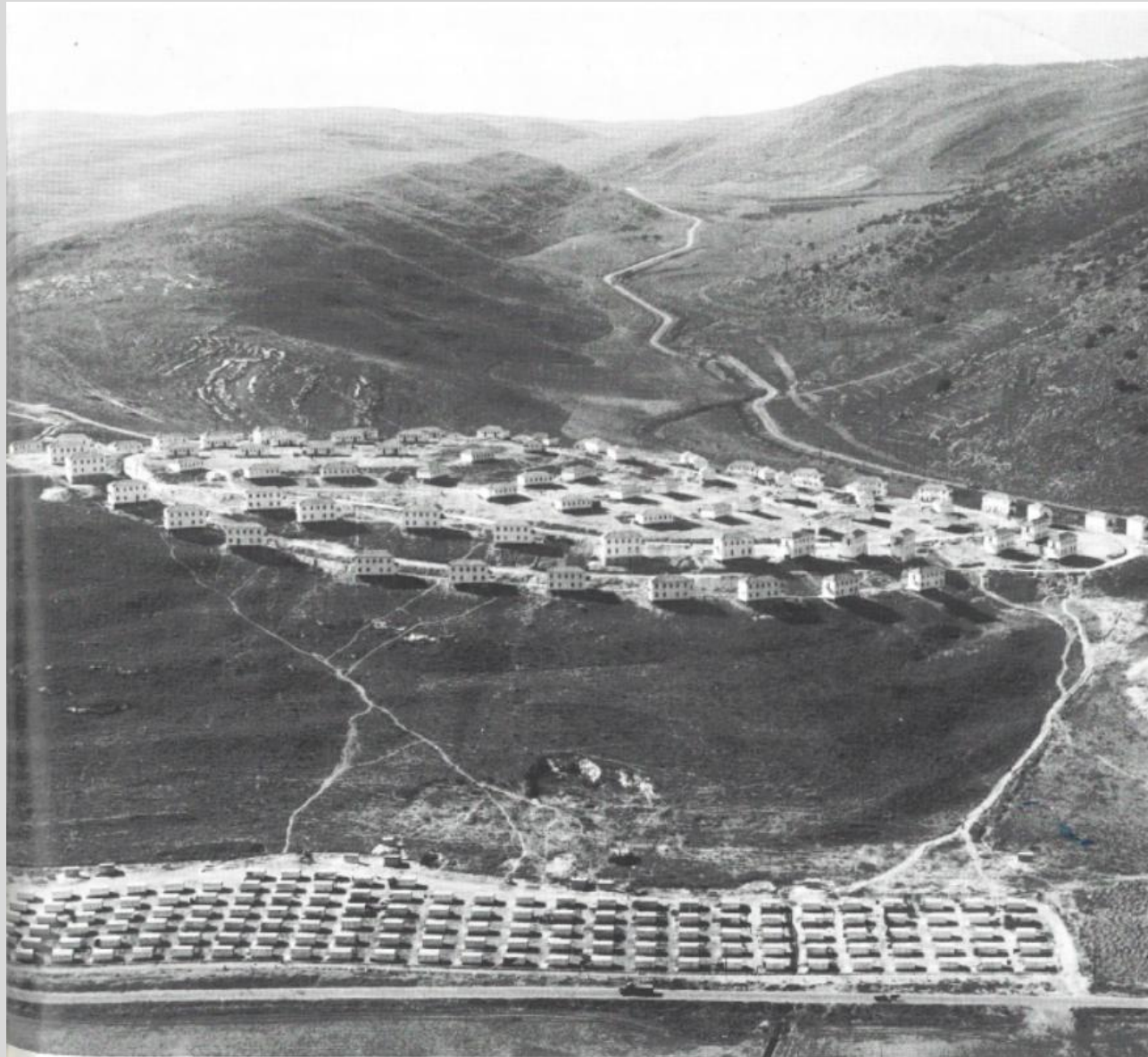
A neighbourhood unit in the new town of Yokna'am, being constructed by the immigrants living in provisional shacks along the road
